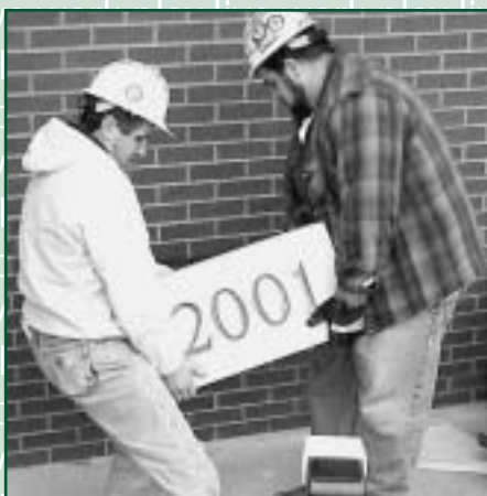
Workers install the cornerstone to the new Stockade Building at Schenectady County Community College. A sealed time capsule with photos, publications and other mementos from 2001 was placed behind the cornerstone to be opened in 2069 on the college's 100th anniversary.
